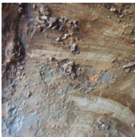
Figure 1. The surface of the carbon steel cooler, after the removal of corrosion products, indicates a progressive degree of corrosion.
